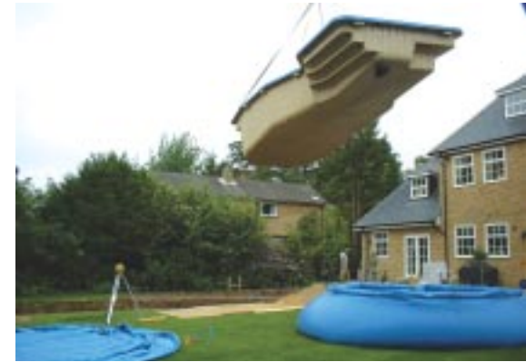
The crane easily lifts the pool from the front over the house.
